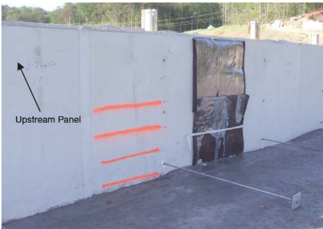
Prefabricated panels covered with a synthetic geomembrane liner were used to waterproof the upstream face of Hickory Log Creek Dam.
