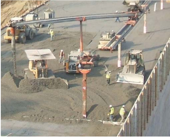
Different sized dozers were used to spread the roller-compacted concrete for Hickory Log Creek Dam. The equipment featured a laser-guided system to obtain a level surface.
