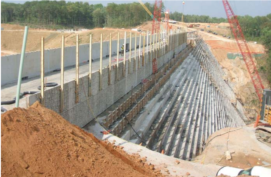
The downstream steps of Hickory Log Creek Dam were formed using grout-enriched roller-compacted concrete (RCC), which provides an improved appearance over typical exposed RCC.
