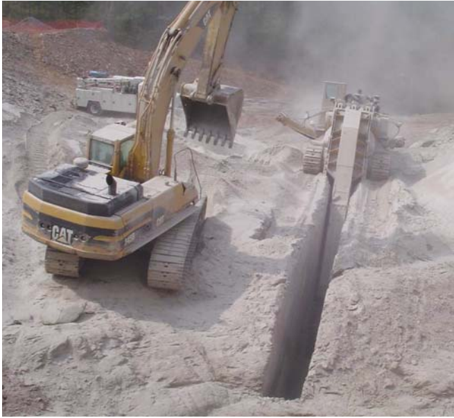
A concrete cutoff wall was built at both ends of the abutments of Hickory Log Creek Dam to provide seepage control.
